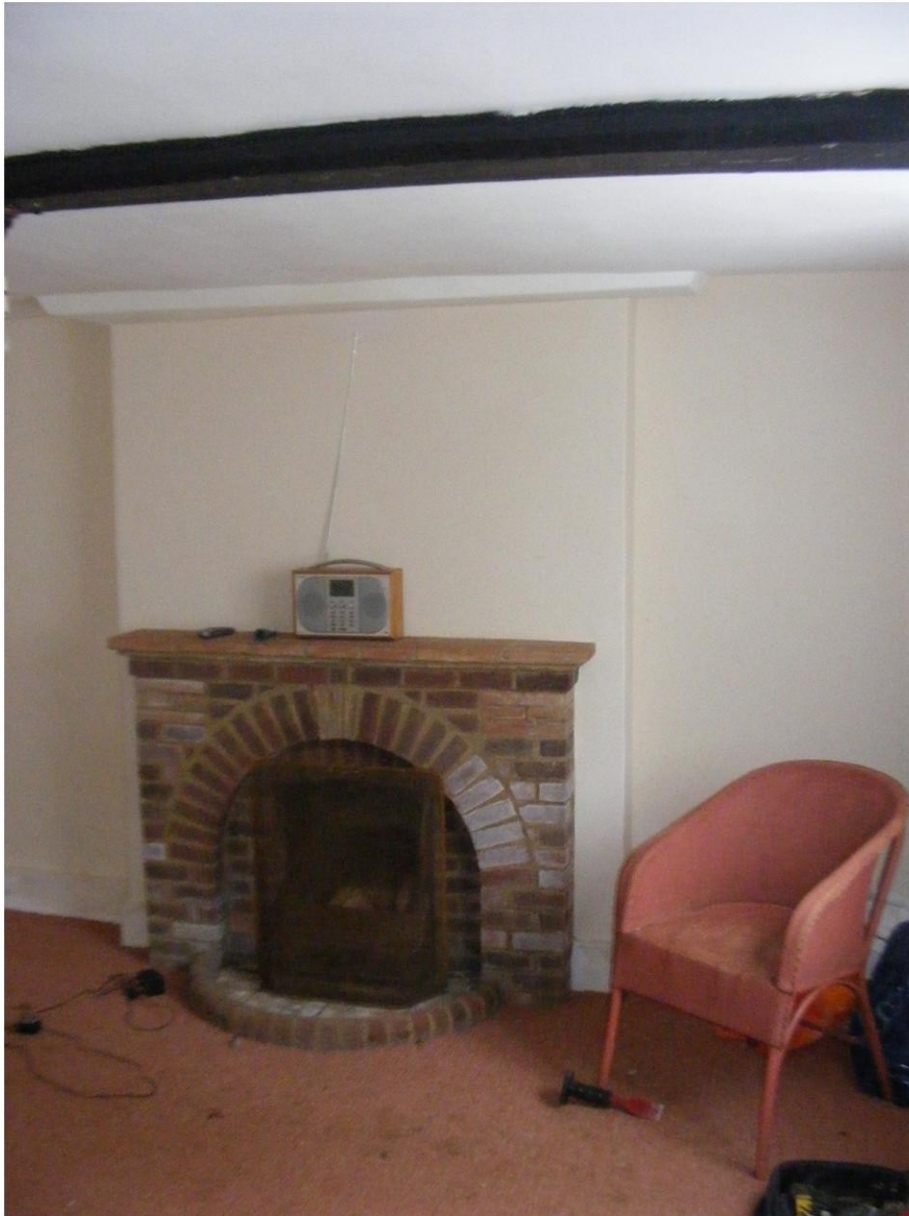
Modern Fireplace in Living Room
