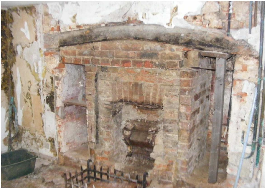
Defective Bressemer Beam and Masonry to Dining Room
