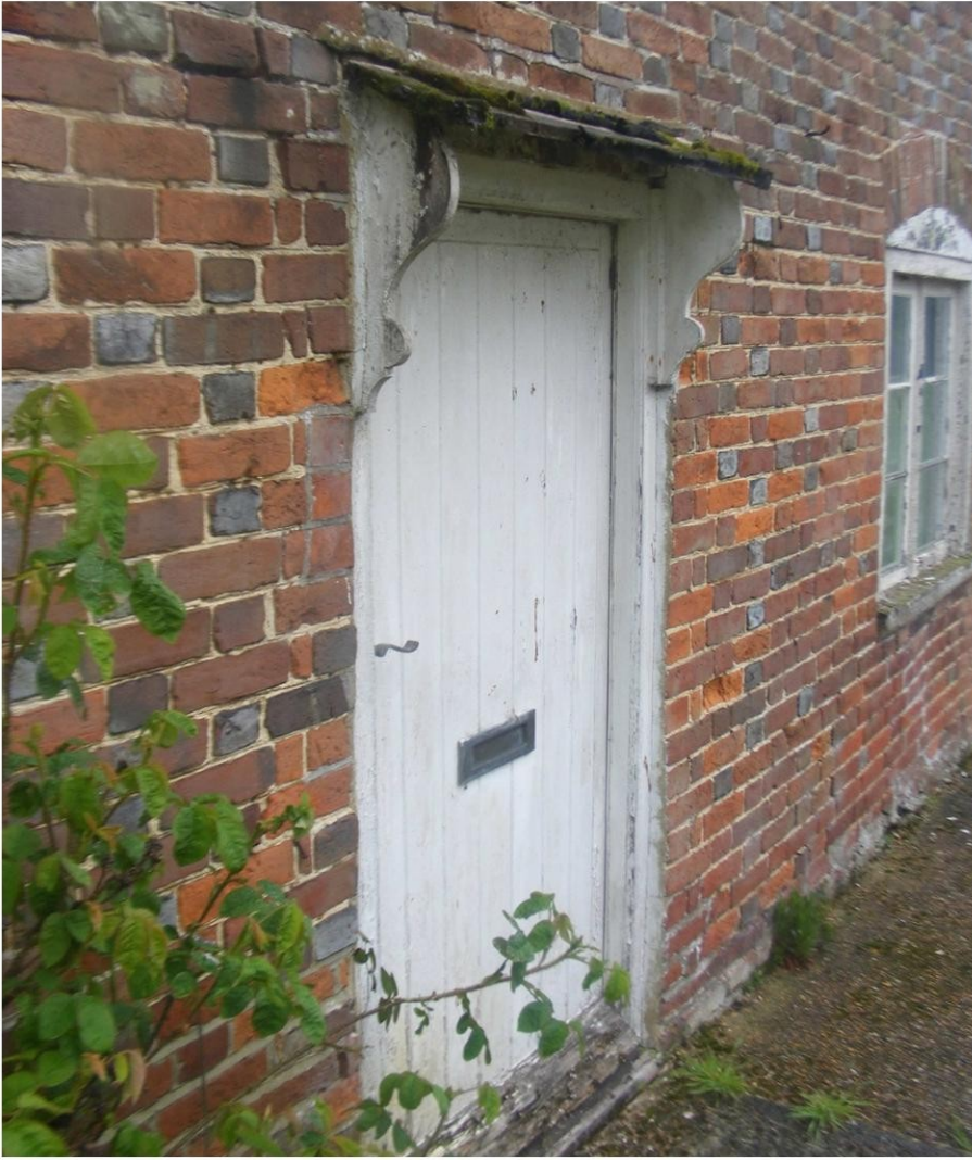
Front Door and Canopy (Poor Condition)
