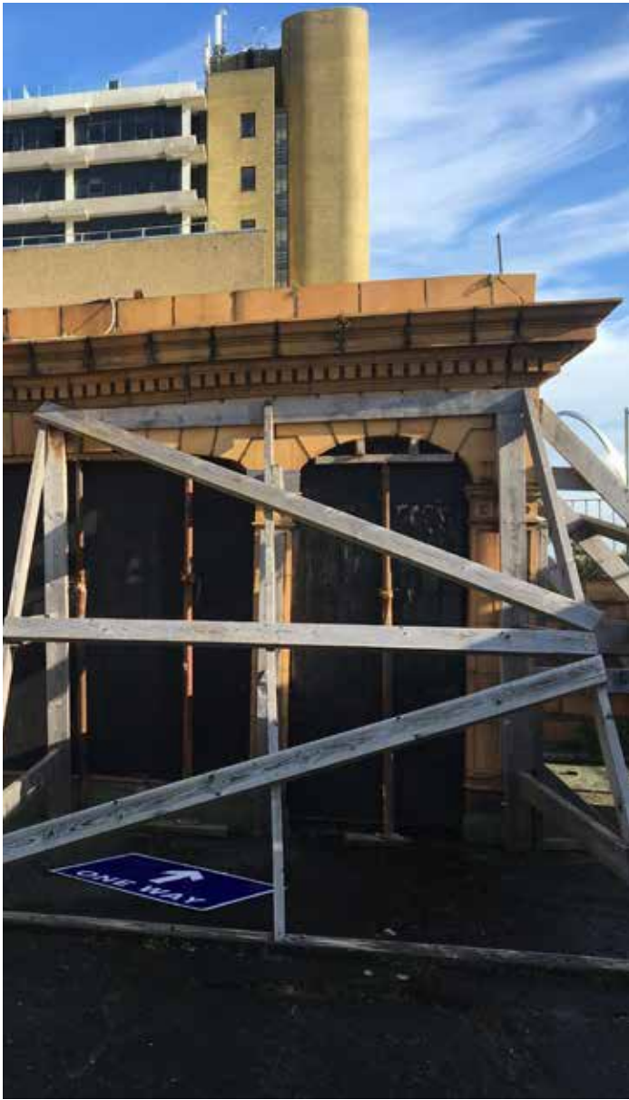
1. The building frontage has suffered serious structural damage. Specialist structural work will be undertaken to stabilise the facades and restore them to their former glory, including the dismantling of the failed southern arches, under the recommendations of the structural engineer and terracotta specialist.
