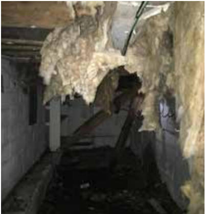
8. The roof of the beer cellar has collapsed.
