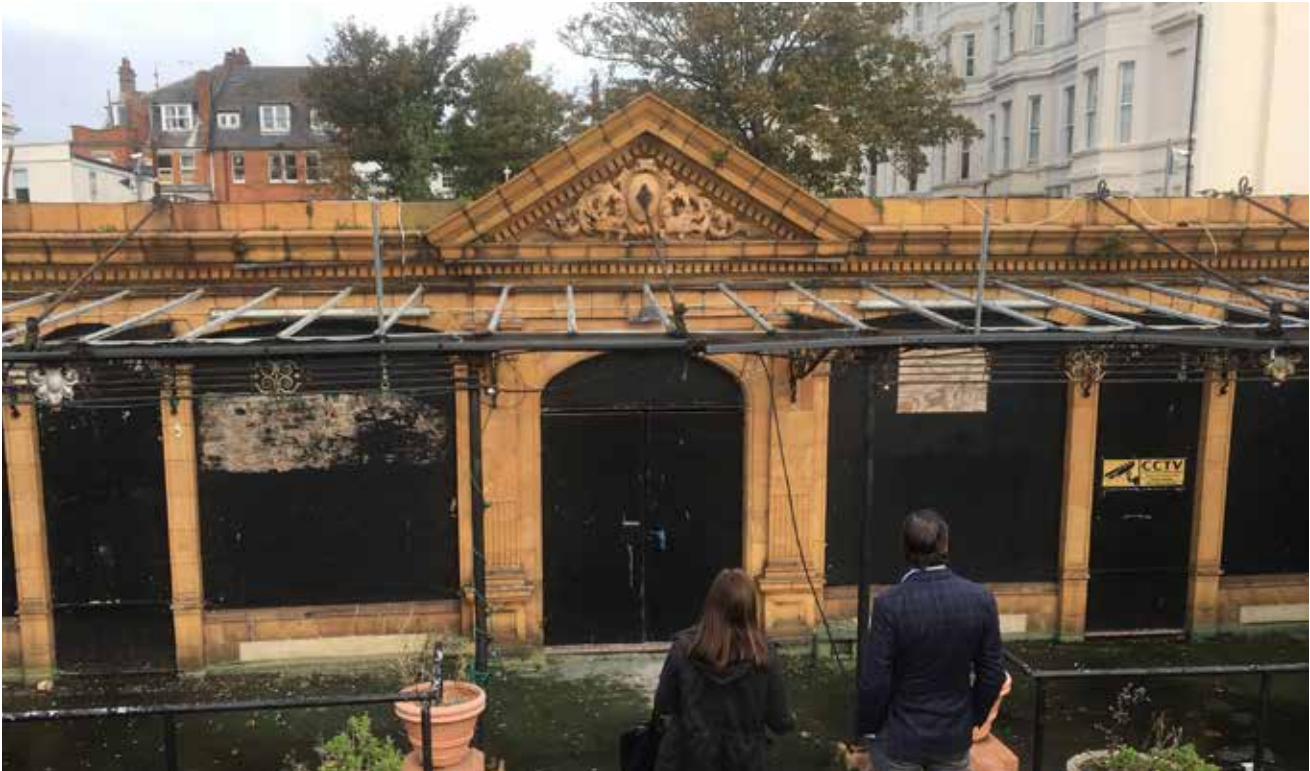
2. The terracotta is damaged in several places and will be sensitively repaired by a terracotta specialist.
