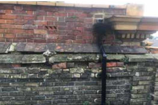
5. The brickwork on the east facade is in need of repair. This will form part of a semi-basement car park.
