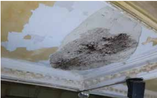
12. Although the main roof is now watertight, the ceiling has been damaged.
