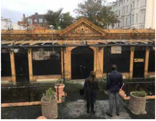
In 2020 the Leas Pavilion has been closed for 10 years. The building is in a state of disrepair and needs renovation.
