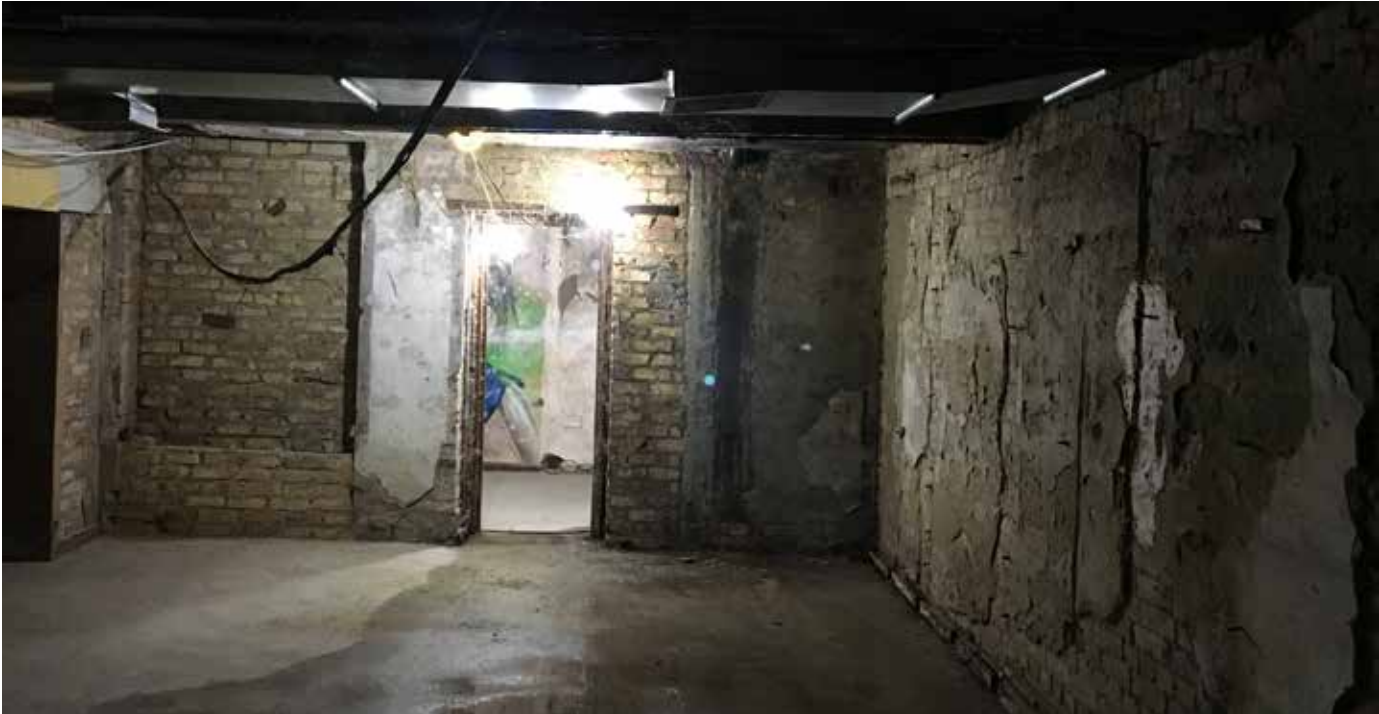
7. Water is leaking into the old bowling alley. Works are required to stop the ingress of water, to ensure the area is structurally sound and to repair and refurbish the space.
