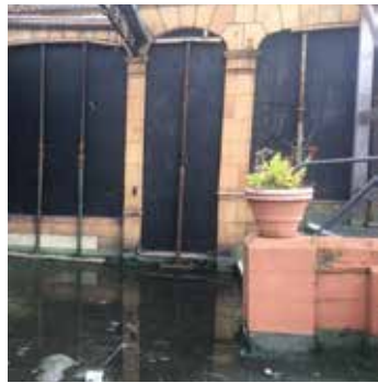
3. The asphalt courtyard has cracked and bubbled. Water gathering in the lower areas is leaking into the basement below. This will be removed and replaced, the structure repaired, and a new waterproof covering laid with a paving finish to be agreed with the conservation officer.
