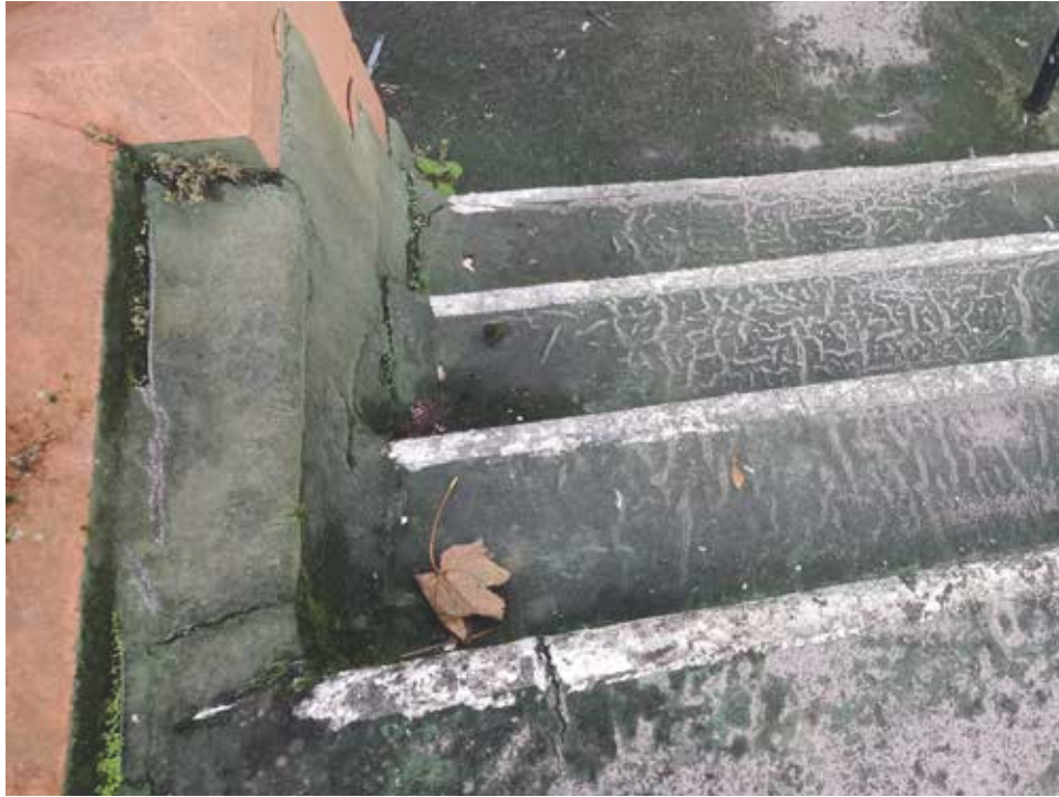
Photo 12: Failing asphalt to external entrance steps
