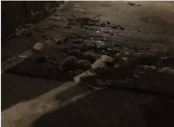
10. The bowling alley is affected by water ingress.
