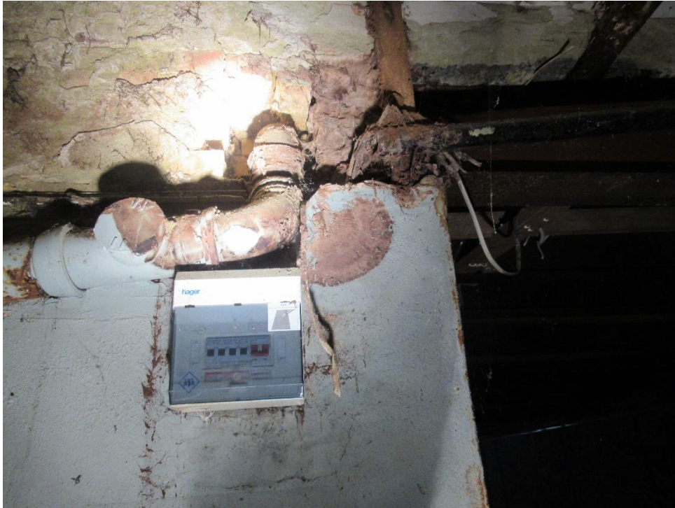
Plate 3. An example of gaps associated with girder and pipework in B1.
