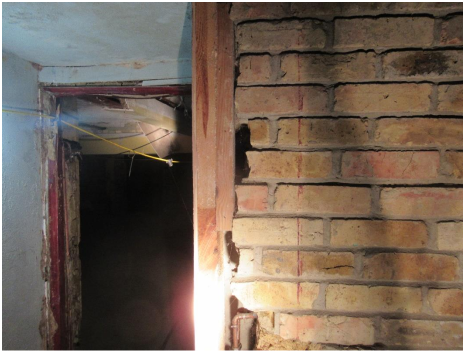
Plate 1. An example of gaps in the brickwork in the 'Bowling Alley' (B1).
