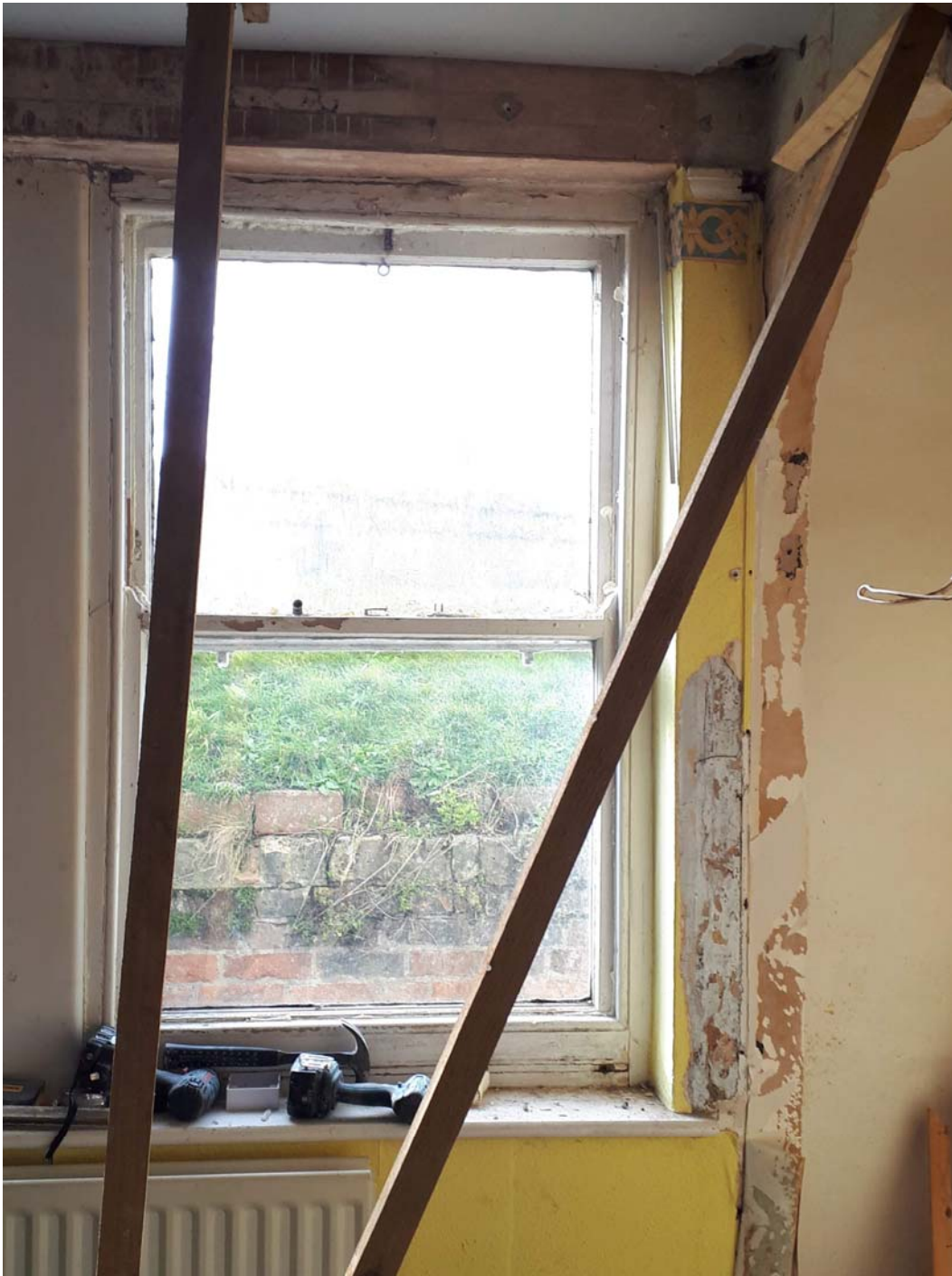
Current windows in poor state of repair
