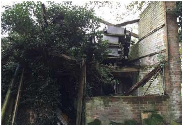
View showing collapsed roof
