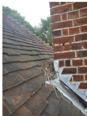
Figure 3: THE DISUSED HERRING GULL NEST BY THE CHIMNEY IN THE MIDDLE OF THE ROOF.
