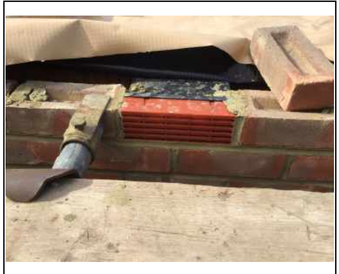
Air brick in place.
