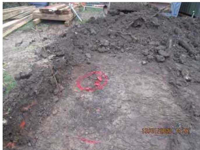
Photo 3 – Example of cement asbestos fragments entrained within Made Ground
