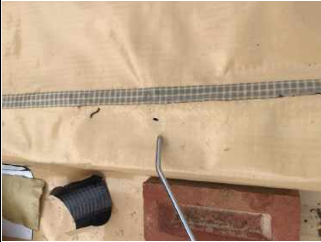
Air lance test finding a defect in the welded joint.
