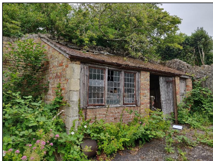
Photo 24: Building B2, dilapidated storage building (photo taken 9 th July 2019)
