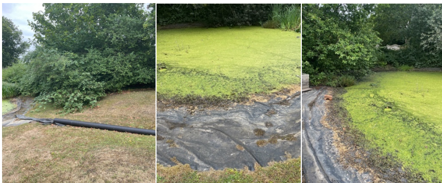
Plastic piping connecting drainage (July 2022)
