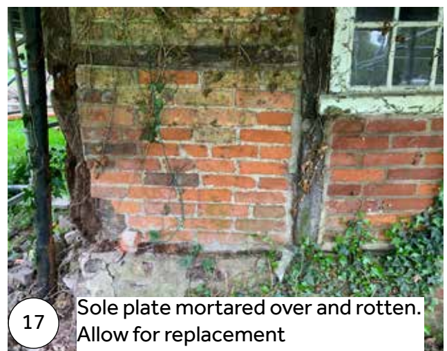
16 Sole plate mortared over and rotten. Allow for replacement
