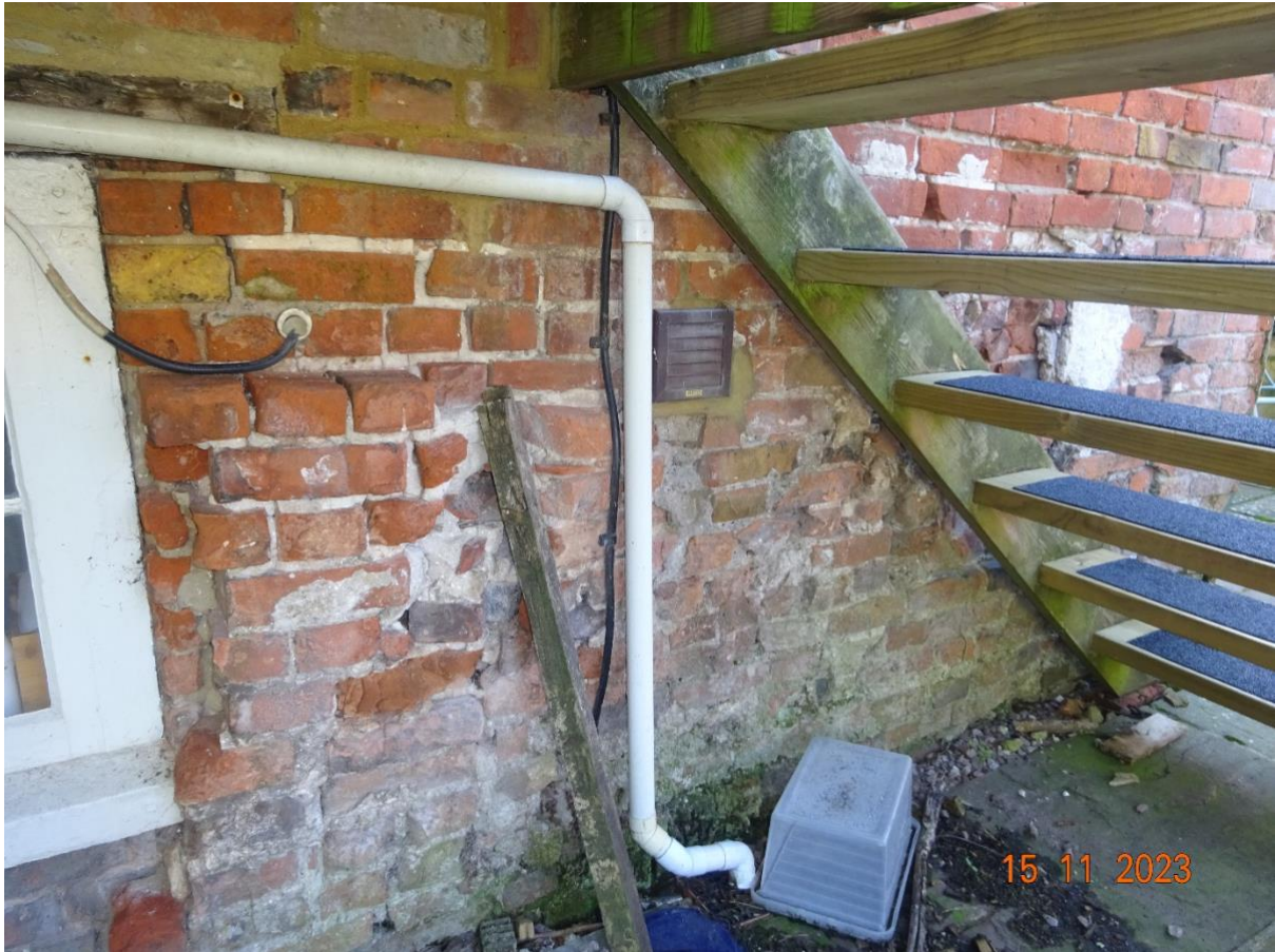
Brickwork on rear of building that needs rendering
