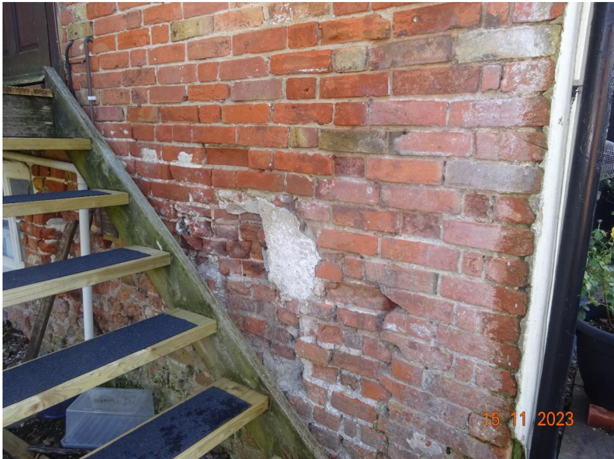
22 High Street, New Romney. Brickwork that needs rendering at the bottom and repointing above – rendering about 800mm from ground so roughly 10 courses up
