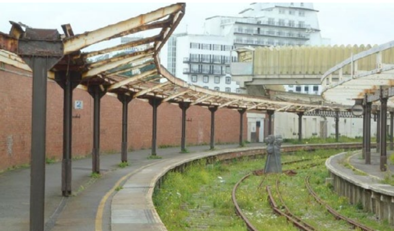
Fig 6.7.2 The dilapidated Harbour Station
