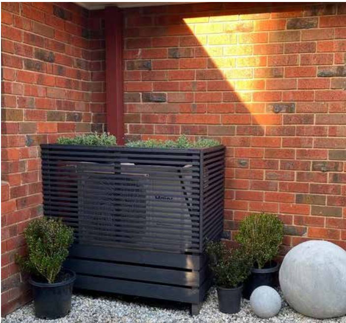
Air Source Heat Pumps
