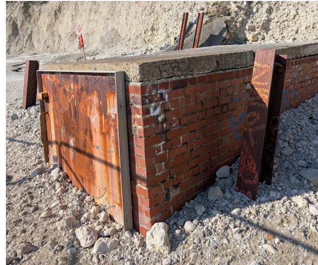
Figure 14. Subsided brick building
