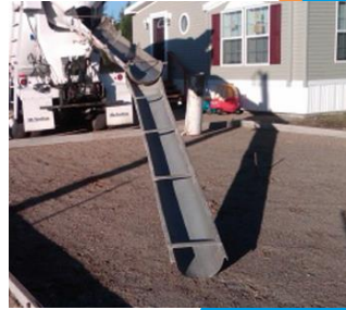
Concrete Chute Extension
