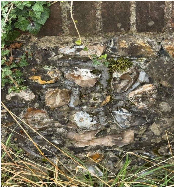
Incorrect pointing of flint (trowel).
